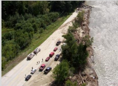
Figure 38: Washed-out roadways in Vermont following Hurricane Irene were restored rapidly to "better than new" condition despite considerable damage.
